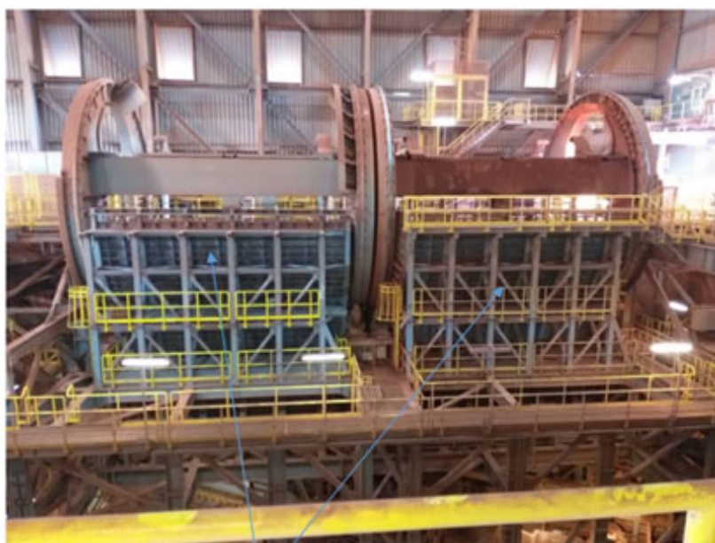
Figure 6-1: New impact walls on Phase 1 and Phase 2 tipplers - February 2020 (indicated by blue arrows)
