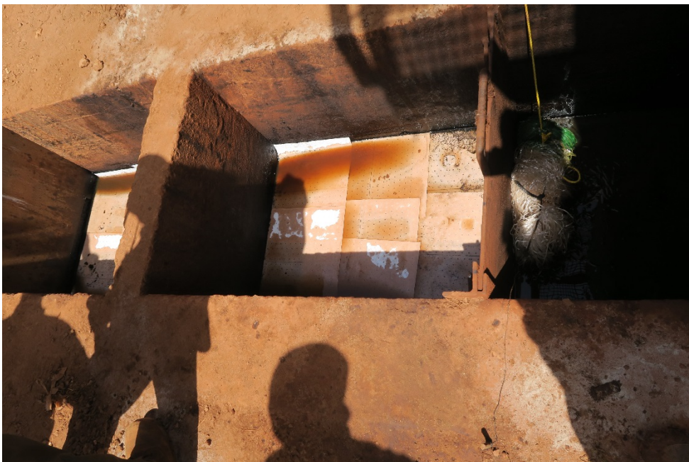
Photo 28. Discharge from the main oil and water separator – note orange discolouration
