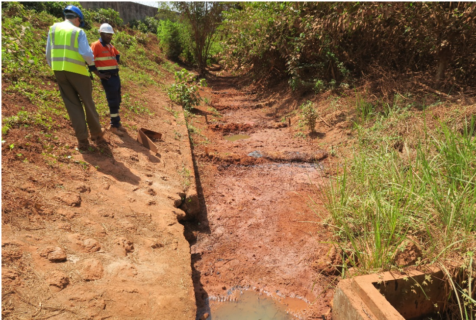
Photo 27. Location of the oil discharge - post clean up
