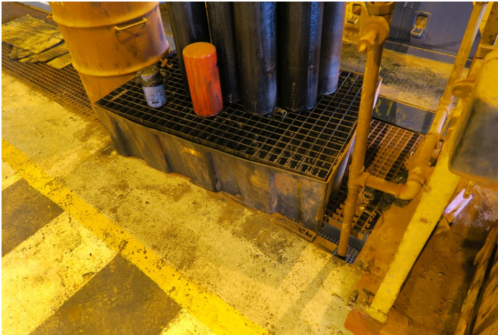
Photo 19. Drip tray used when draining filters – full to capacity
