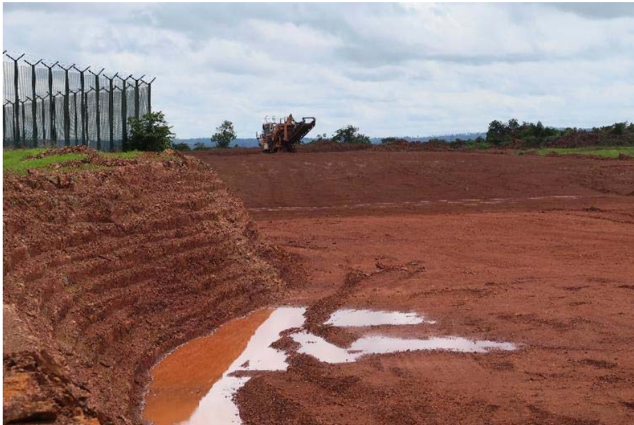
Photo 4. Surface miner – note creation of steep and unstable mine face
