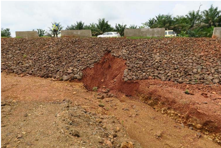
Photo 16. Recently completed section of COBAD Road – erosion and damage to rock armoured slopes
