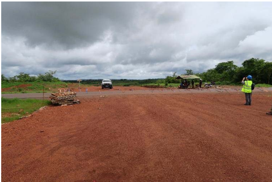
Photo 12. Crossing of COBAD Road and the main road between Boke and Sangaredi (N3) – no overpass/underpass as referenced in the ESIA
