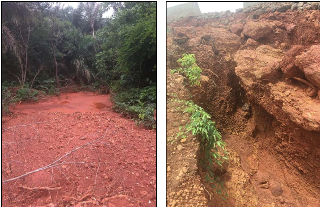
Figure 10-4: Left – large area of sedimentation and run-off from COBAD road in gallery forest critical habitat, right – two-metre deep eroded pit in COBAD road drainage ditch
