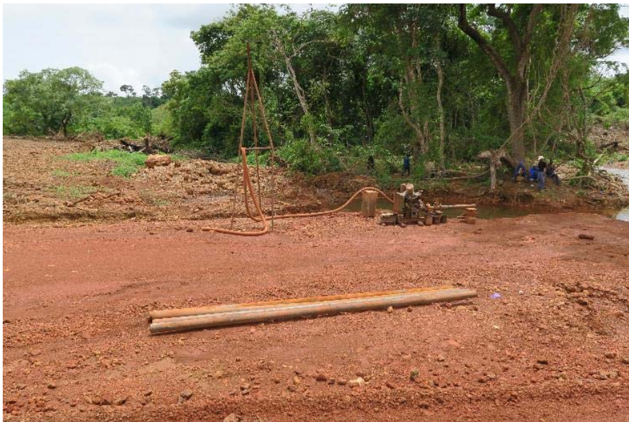
Photo 14. COBAD Road – abstraction of surface water contrary to mitigation measures specified in the ESIA
