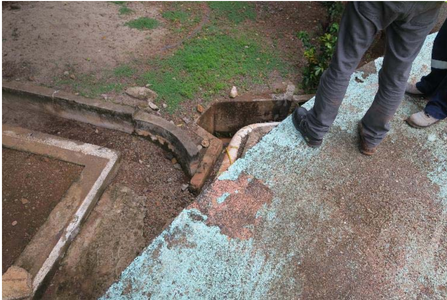
Photo 7. Unprotected raised platform at water treatment plant – fall risk
