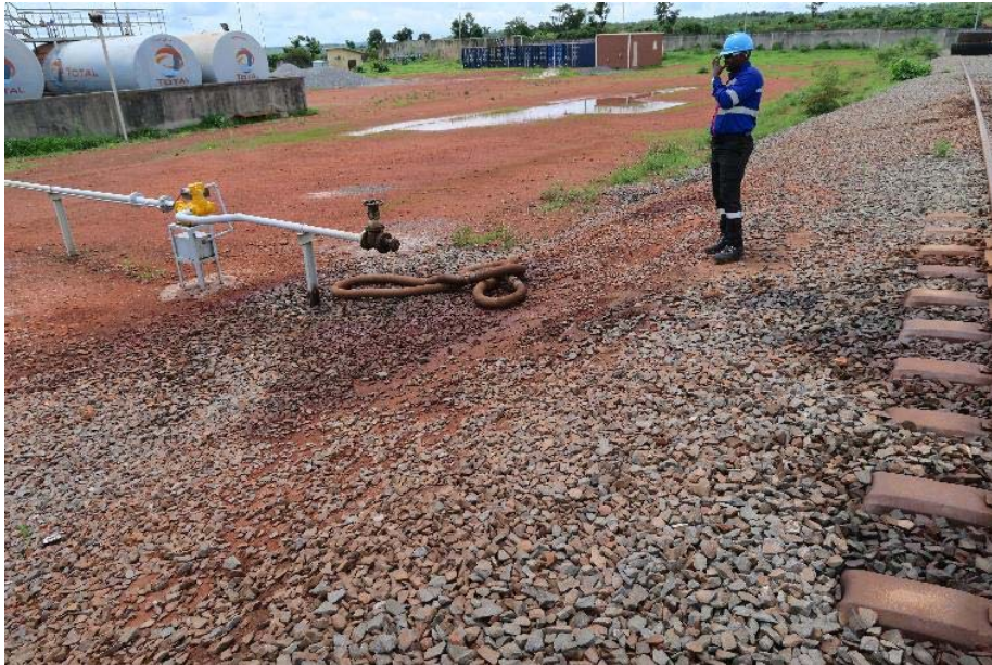
Photo 5. Fuel spillages at Sangaredi power plant – same spillages observed in November 2016
