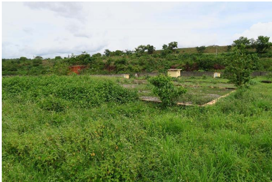
Photo 10. Waste water treatment plant at Sangaredi – overgrown (inefficient) filtration beds
