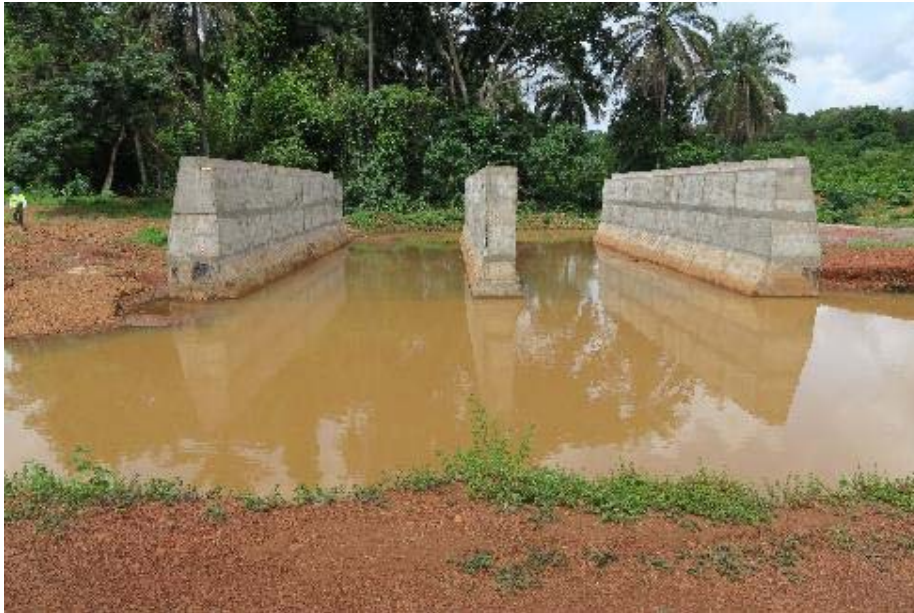
Photo 19. Part constructed bridge on the abandoned section of the COBAD Road – no progress since Nov 2016 visit
