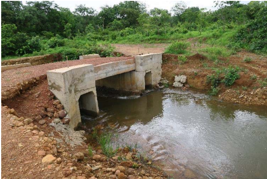
Photo 21. Significant erosion around bridge – wooden planks required to cross bridge on the far side following erosion
