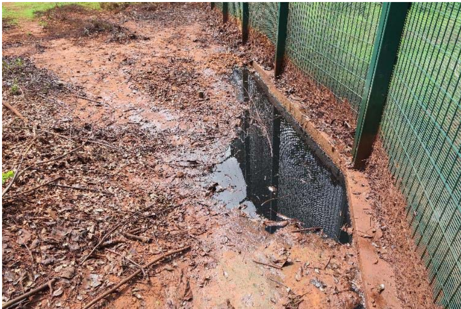
Photo 2. Sangaredi maintenance workshops – pooled oil at discharge location on the site boundary
