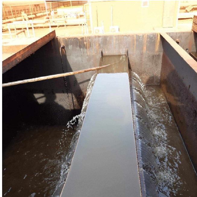
Photo 30. Oil water separator – treated water
