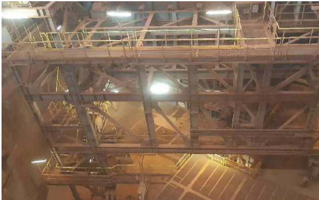
Photo 22. Evidence of fallen rocks. IESC understands no personnel are allowed access whilst tippler is operational
