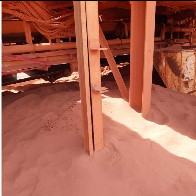
Photo 25. Accumulated dust beneath conveyors/moving machinery at Kamsar
