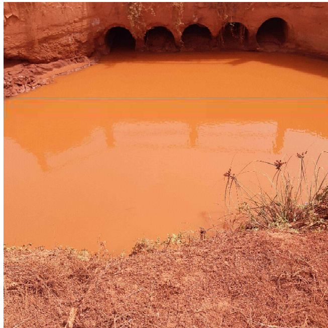
Photo 24. Heavily sediment laden discharge exiting CBG perimeter.
