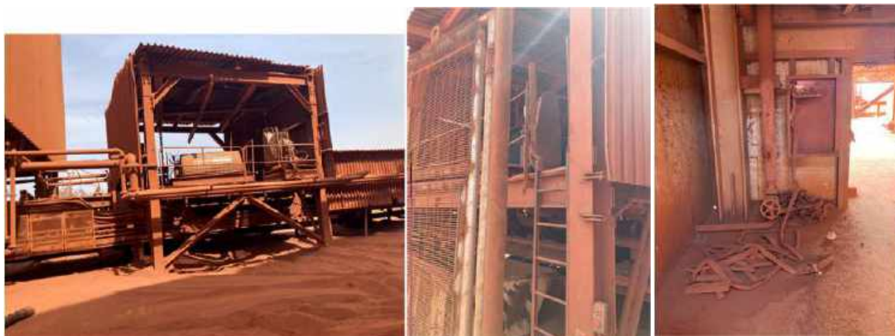
Figure 6-1 “Déferailleur”(Carter Missing or Defective) and Fire Hoses Broken on the Floor
