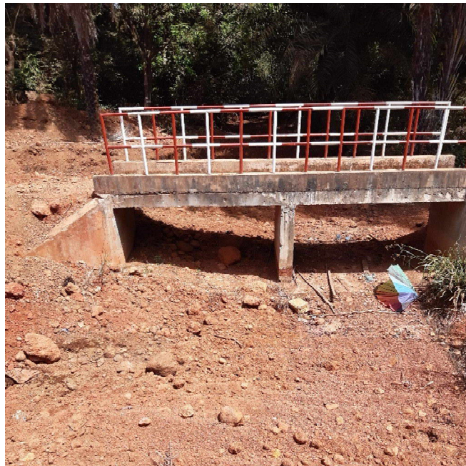
Photo 10. Poor construction practice adjacent to dried up stream. Earthworks resulting in soil being moved into the dry stream
