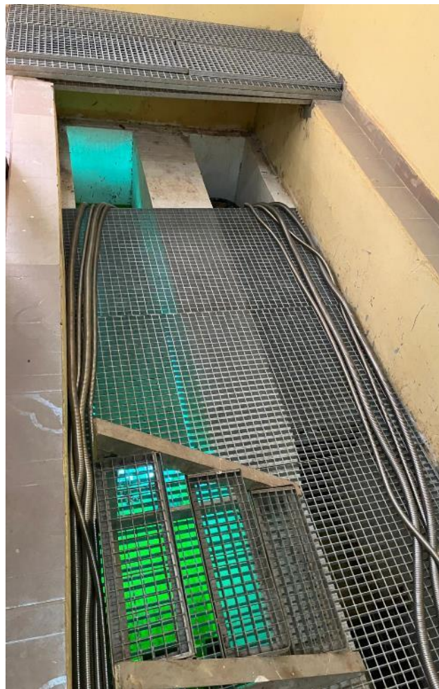
Figure 8.2 The UV treatment at Sangarédi WWTP (under operation)
